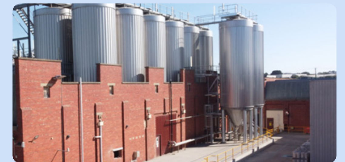
Brewery tanks at Little Creatures Geelong
